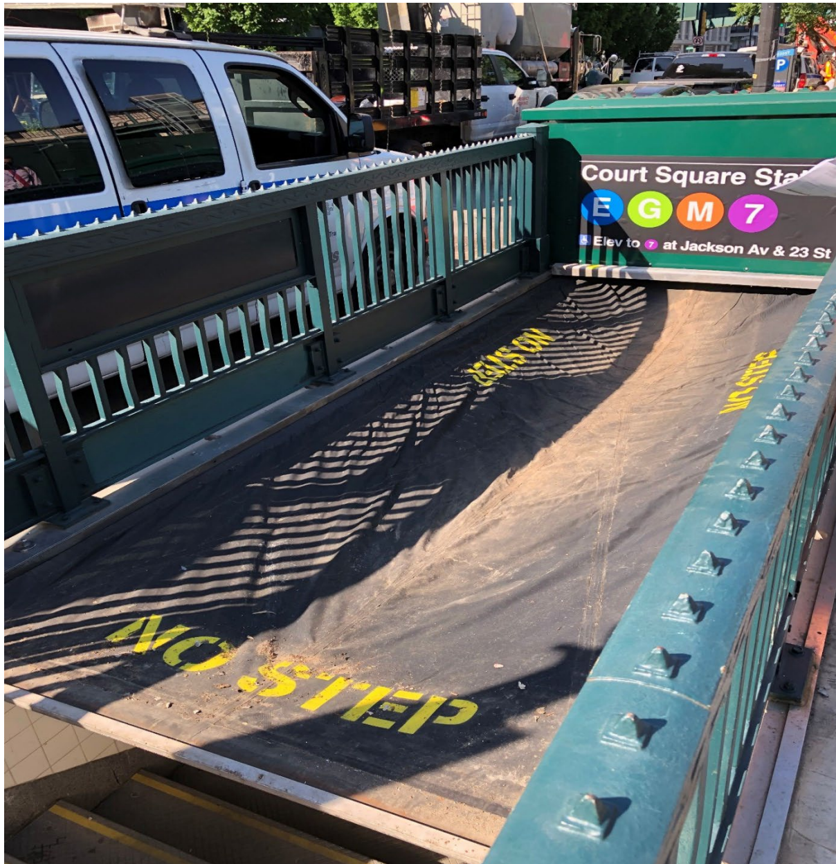
Partially closed flex gate at Court Square Station
