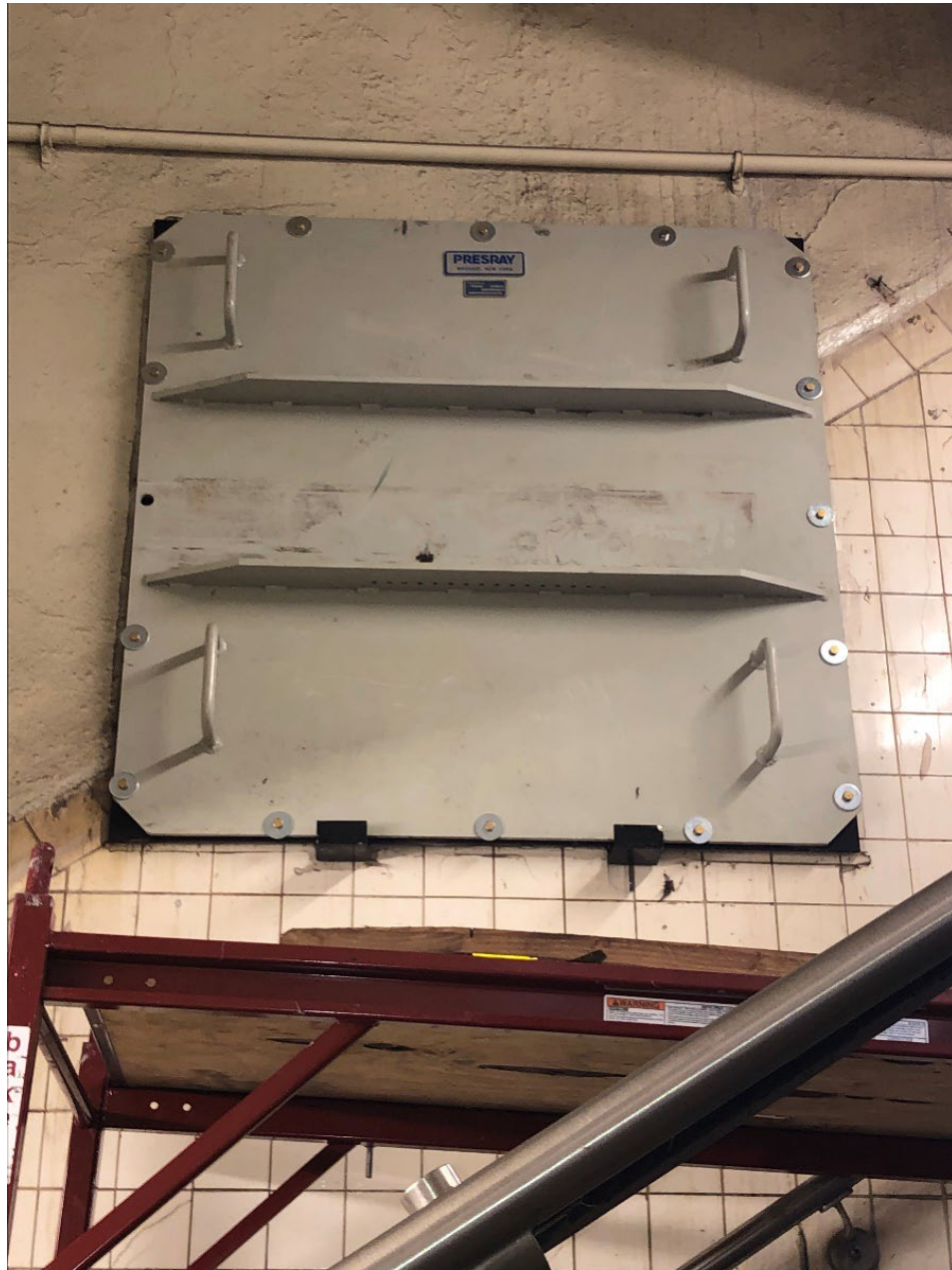
Watertight hatch covering wall vent in station stairwell, Vernon Boulevard–Jackson Avenue Station
