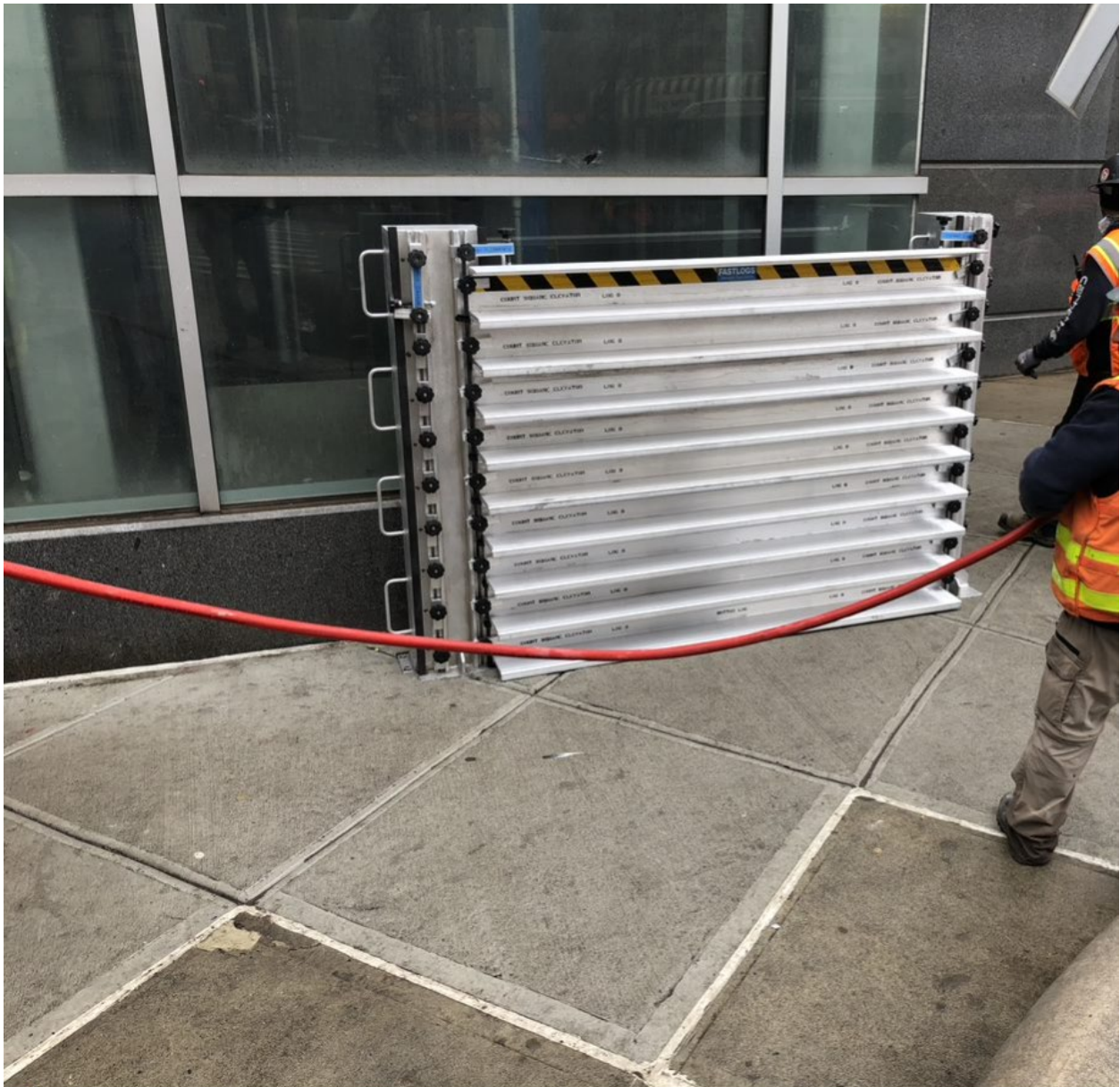
Section of stop logs protecting side of Court Square Station elevator, moments before spray test
