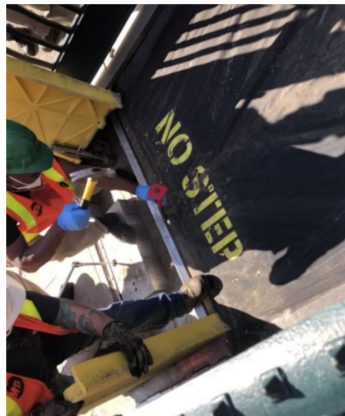
Workers trying to deploy a flex gate with a hammer and chisel, which could damage the membrane.
