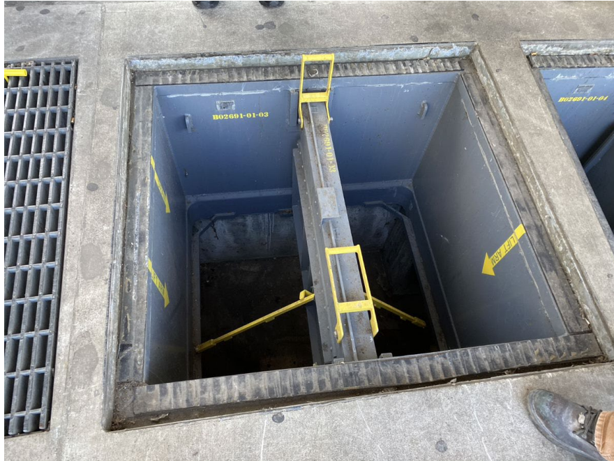
MCD in the “open” position at South Ferry
