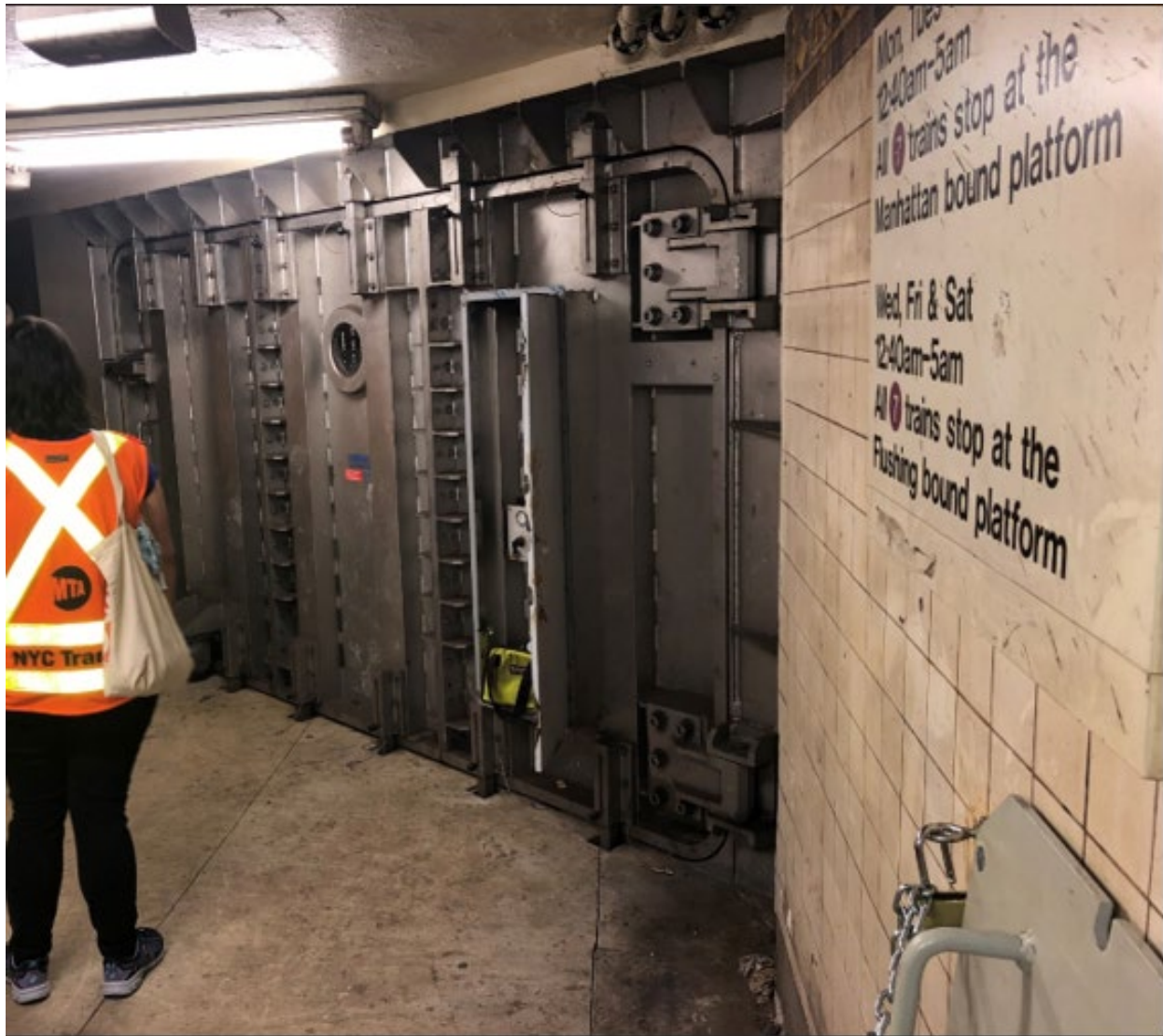
Activated marine door at Vernon Boulevard–Jackson Avenue Station
