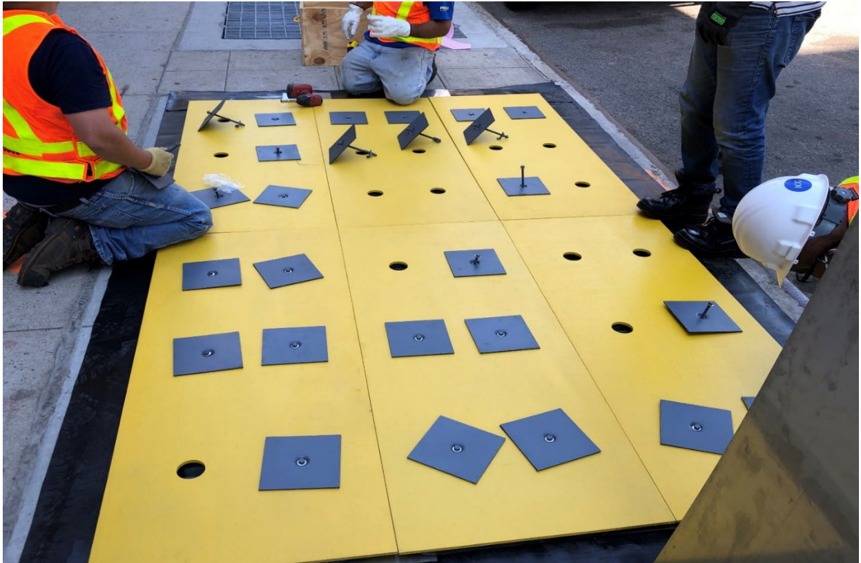
Flood covers over vents at Court Square Station
