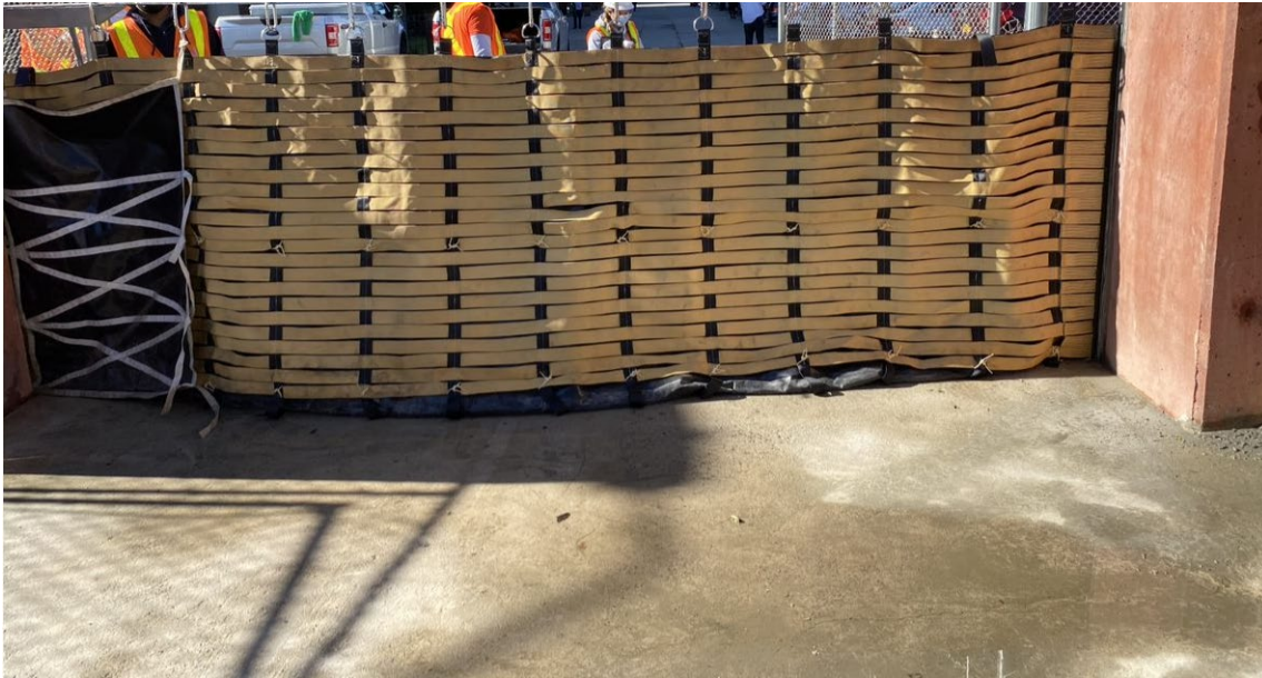
Side deployment flex gate at 148 th Street Yard entrance
