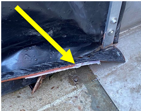
Silicone observed applied to flex gate during water leak test.
