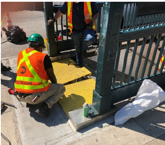
Crew could not re-close a steel plate after flex gate deployment.
